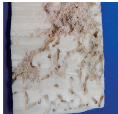
Fig. 20 Heat insulating material damaged by termites
