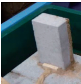
Fig. 9 Mud tubes built on untreated concrete block in one week after installation
