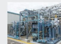
Pilot facility for producing methanol from CO2
