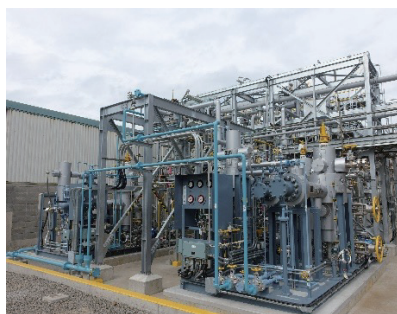
Pilot Facility for Methanol Production from CO 2
