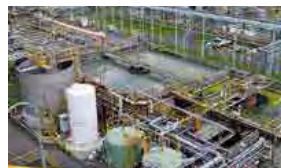
Activated Sludge Treatment Facility
