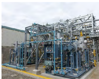
Pilot Facility for Methanol Production from CO 2
