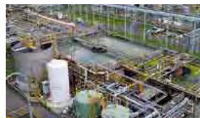
Activated Sludge Treatment Facility
