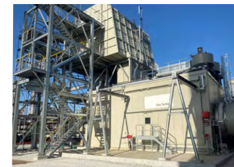
Chiba Works' Highly Efficient Gas Turbine Power Generation Equipment
